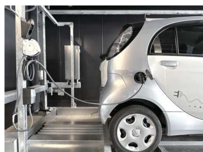
EV charging facility installation and charging management service
